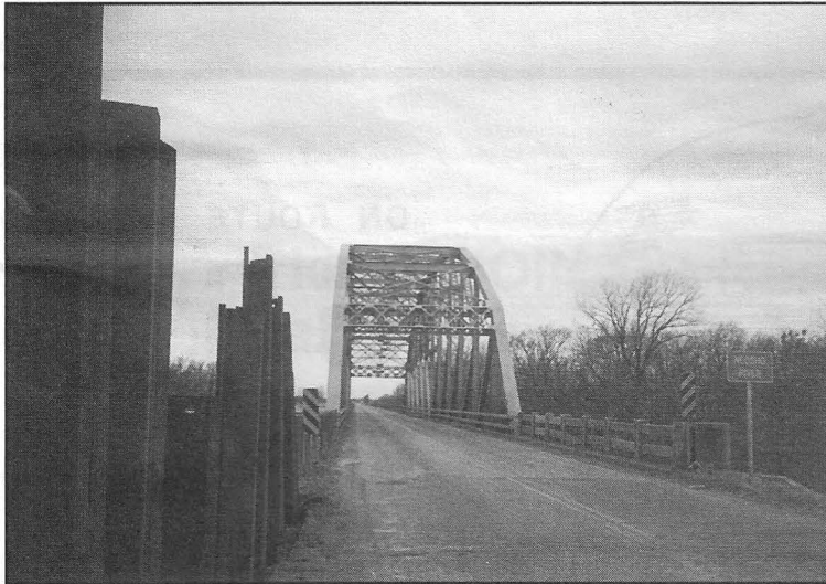
Neosho River Bridge, Miami. New bridge construction to the South side of bridge is already underway.
