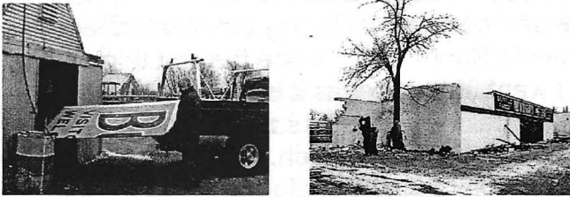
Left: David Kane and Ron McCoy load up the Buffalo Ranch sign. Right: demolition underway.
